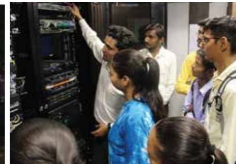
BSNL Ahmedabad Networking & Telecommunication server room
